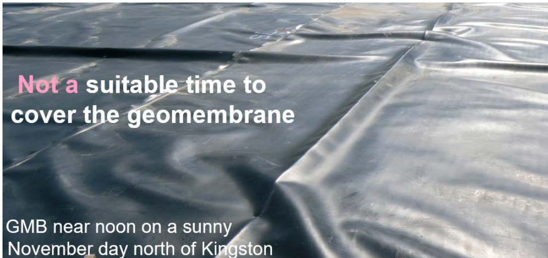
Figure 3: To minimize/prevent leakage, the geomembrane should not be covered with protection soil with the wrinkling shown. The contractor would be required by the CQA consultant to defer covering until wrinkling decreases to a negligible level (e.g., Figure 4)
