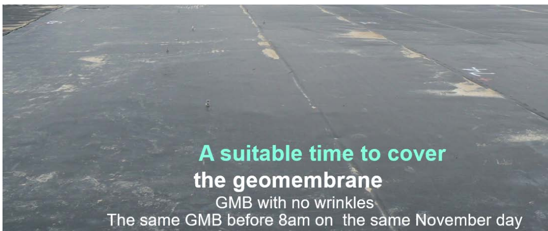
Figure 4: No wrinkles. The geomembrane can be covered with protection soil at this time.
