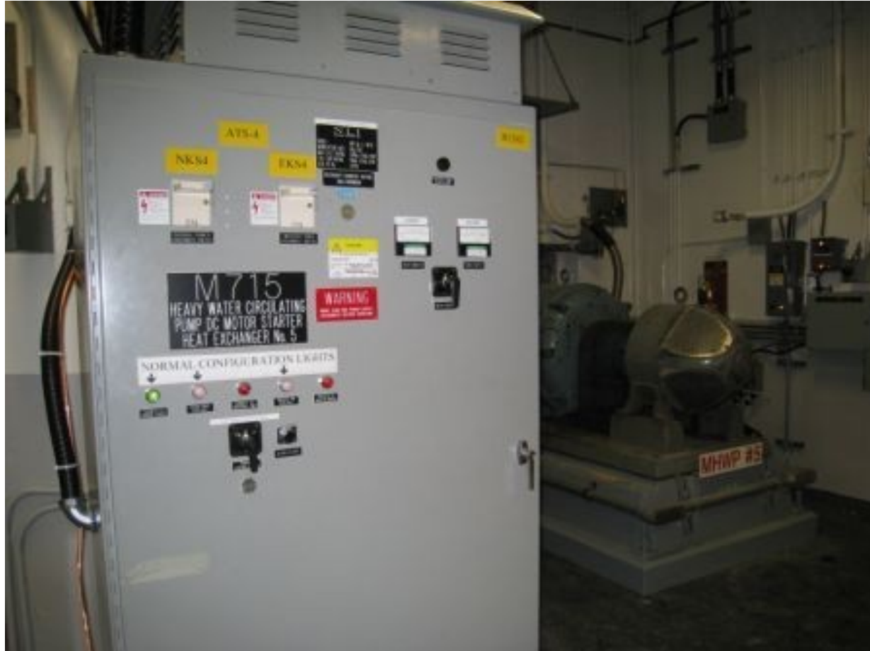
DC Motor Starter For MHWP #5
